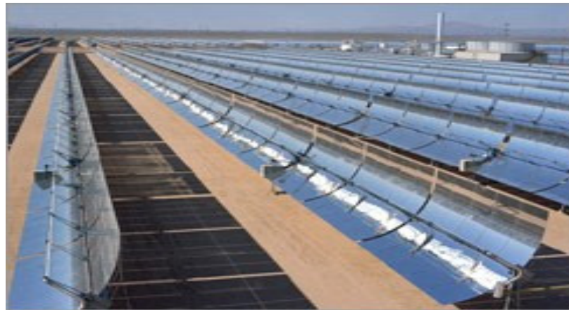
Figure 6. Parabolic Collector of the Power Plant.
