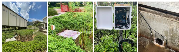
Figure 8 Field implementation of the water level monitoring system in NIE rain garden in NTU, Singapore. One water level LCS, one water level TS and one temperature LCS were installed in the outlet sump.
