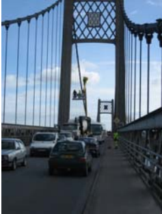
Figure 4: One-shot expensive sensors installation on a structure.
