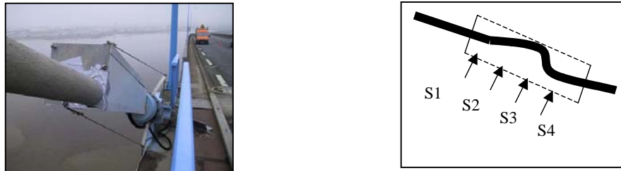
Figure 1. (A) Real-time monitoring of cable anchoring. (B) Distribution of 4 wireless sensors
