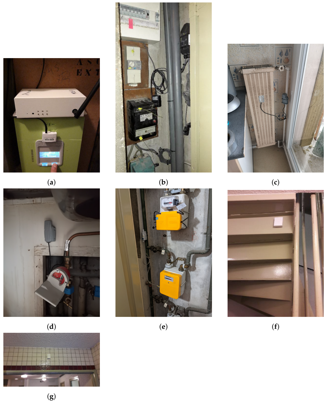
Figure 3. Installed sensors. (a) Pulse sensor installed on a Linky smart meter. (b) Sensor with clamp ammeters for submetering on an electrical switchboard. (c) Temperature sensor for heater surface temperature in apartments. (d) Temperature sensor for DHW pipe temperature. (e) Pulse sensor for a natural gas Gazpar smart meter. (f) Temperature and humidity sensors installed in shared building areas. (g) Presence detection sensor.
