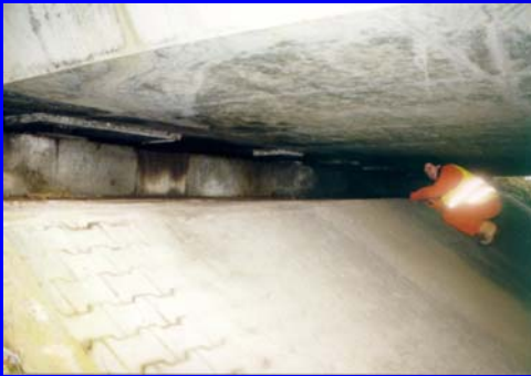
Difficult to access
