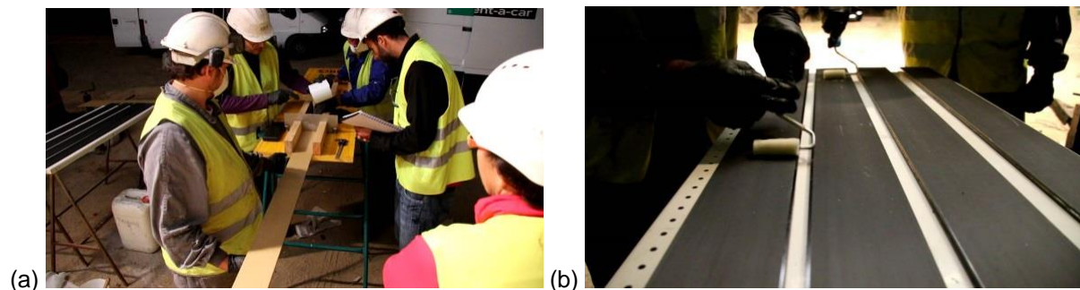
Fig. 3 – CFRP preparation: (a) Application of the adhesive layer and (b) pressure application
