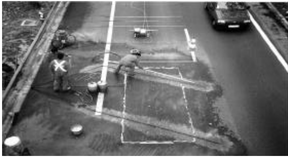
sensor installation on NR 10 (France)
