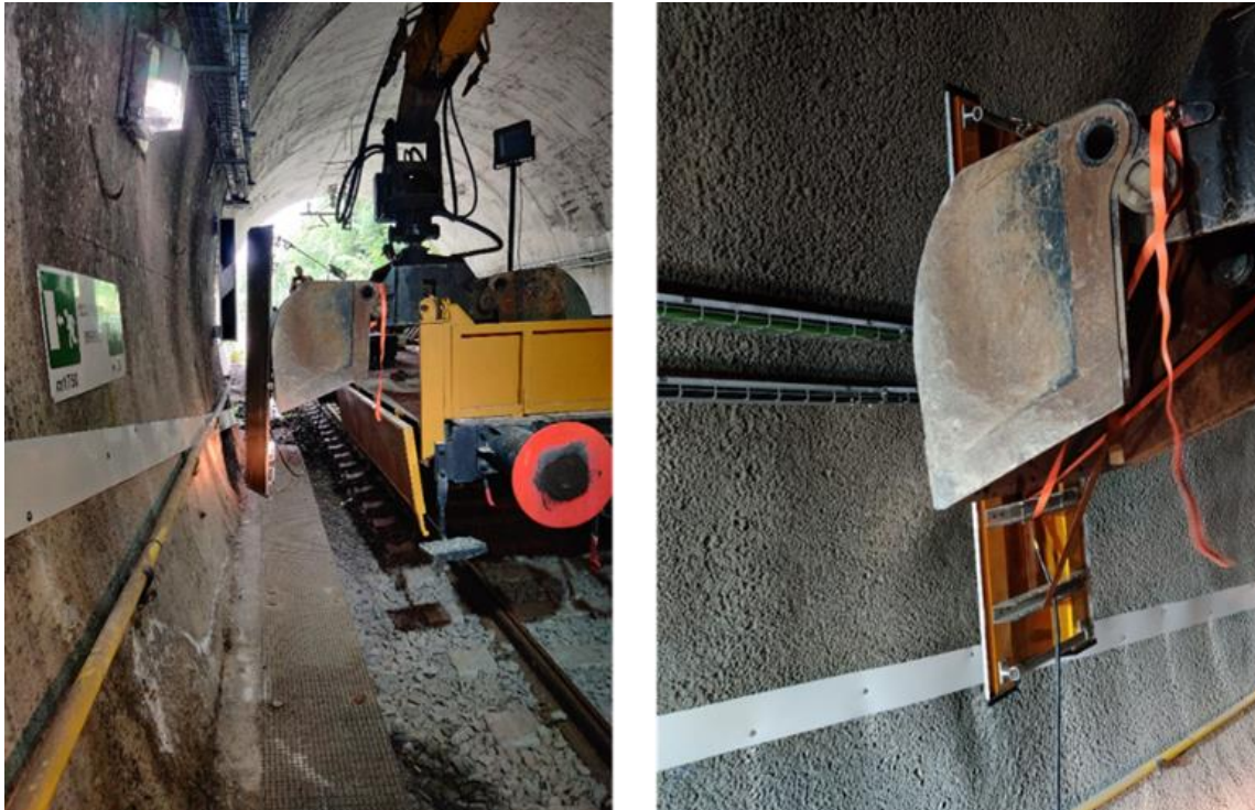
Figure 33. The GPR antenna DX1821 from 3D-radar attached to a shovel of an excavator on the flatcar (Silvast et al., 2021).
