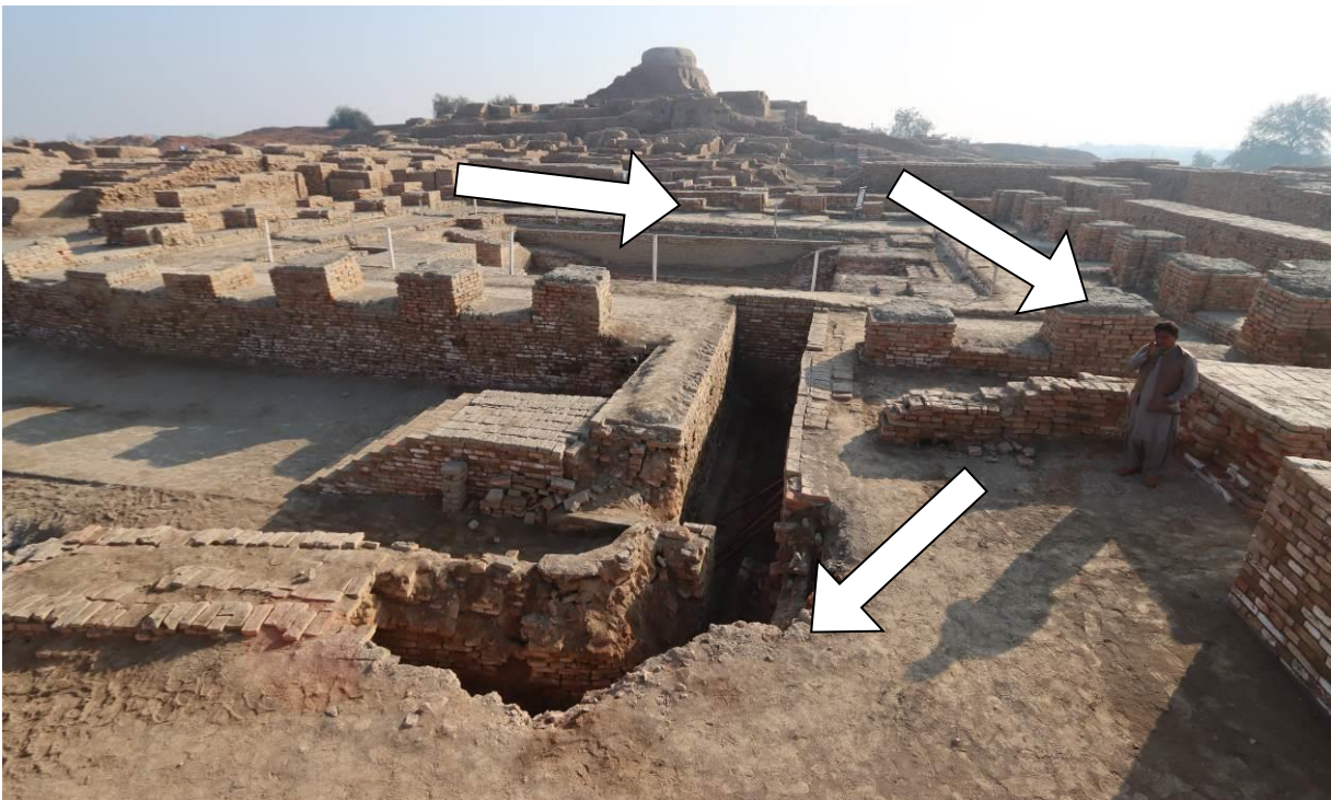
Arrows show the starting point of the collection of water and how run-off has made its way towards the damaged structure.
