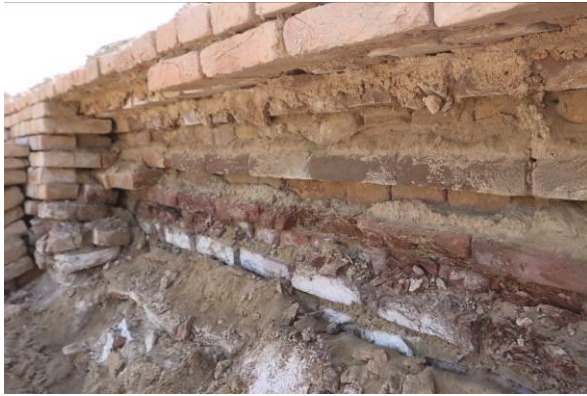
Salt inside the wall visible after collapse, HR Area
