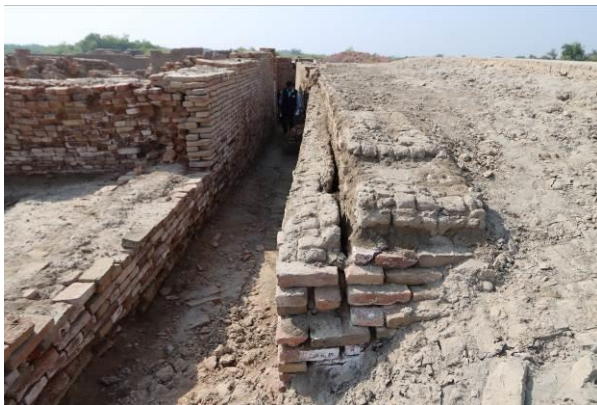
Typical wall deformation with crack at DK Area
