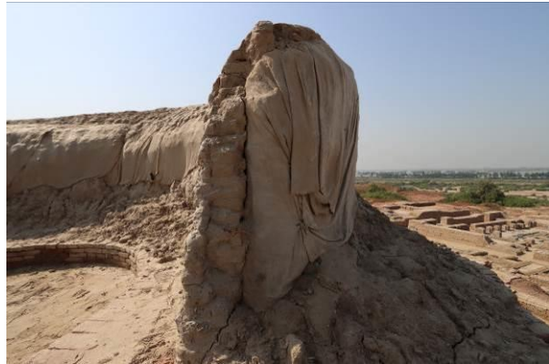
Picture showing fallen part and protective geotextile
