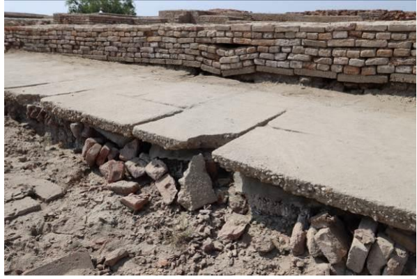
Slopes of pathway led to self and wall damages (L area)
