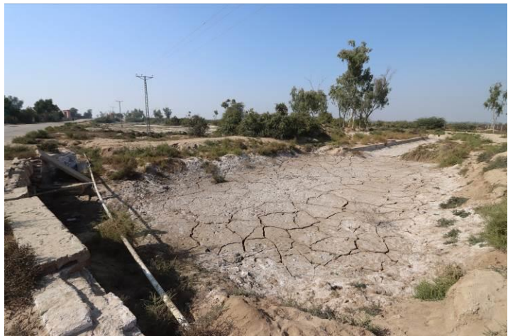
Circular canal exit, blocked by sediments showing presence of salt
