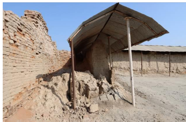
The fallen part (south west end)
