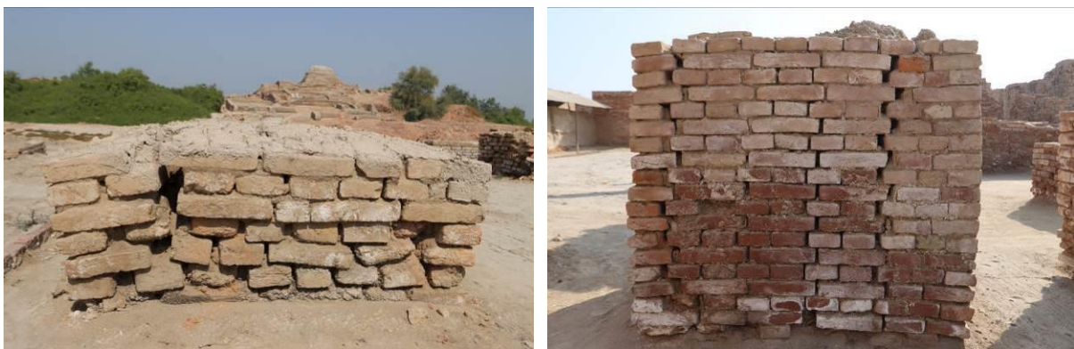
Two column types of wall (L and DKG areas) illustrating well the typical collapse process starting from the base
