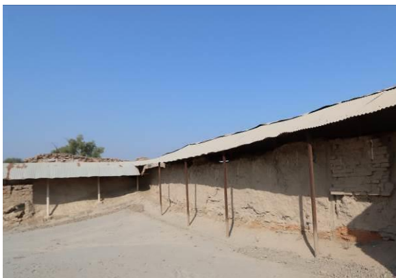
Overall protected wall (fallen part at the left)
