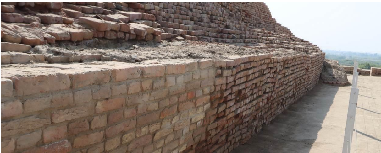
The retaining wall at the base of the stupa (west side) is clearly leaning out
