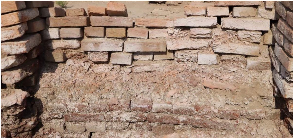
The variety of quality of burnt bricks is very visible on this wall at DKG area, very good state at the base, almost fully disintegrated in the middle, acceptable at the top
