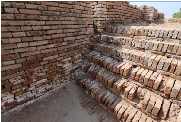
Presence of salts at DK Area
