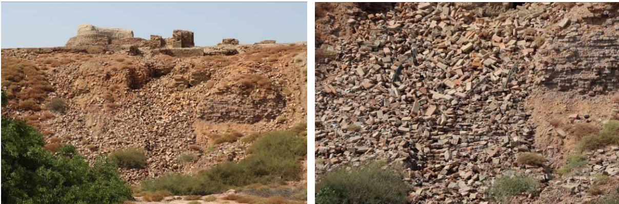
On the eastern side of the citadel area, the huge flows of water collected by the upper platform have revealed some structural elements which could be the original steps to the stupa.
