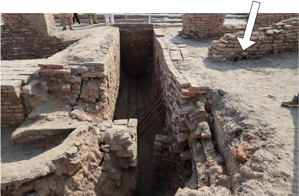
Instability of retaining wall at the southern side of canal from bath in SD area originates from drainage system.
