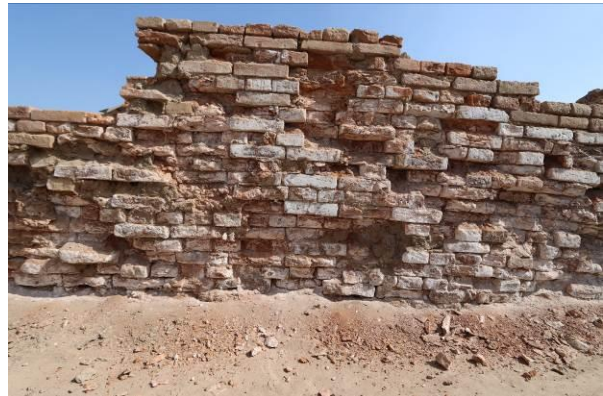
Loss and fall of pieces of fabric due to expansion
