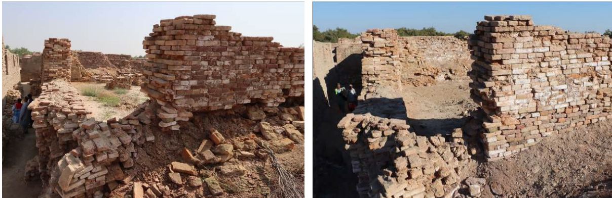
Demonstration of wall base treated temporarily with dry brick wall (without mortar)
