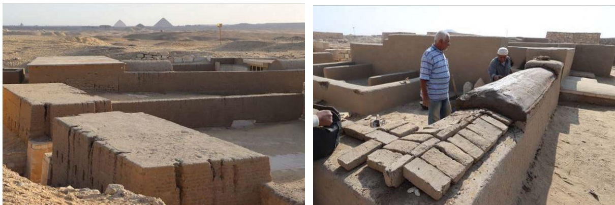
Left: Typical degradation process (formation of gullies) at Saqqara Right : proposed solution for capping (Pepy 1st site)
