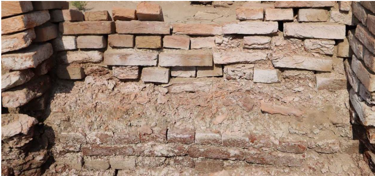
One of the examples discussed: the variety of quality of burnt bricks is very visible on this wall at DKG area, very good state at the base, almost fully disintegrated in the middle, acceptable at the top
