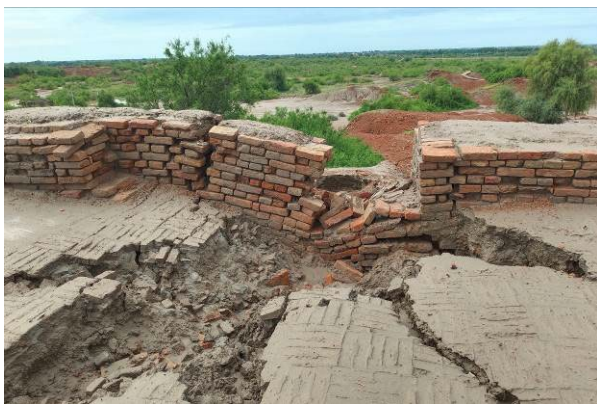
Failure of drainage system at SD area © N. A. Sangha:
