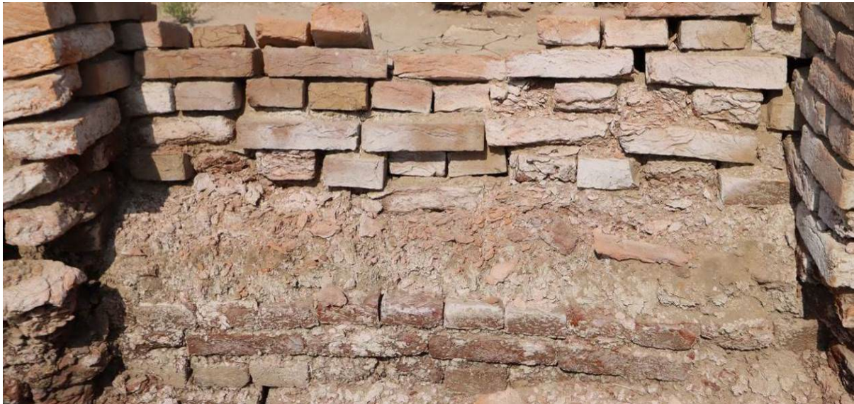
One of the examples discussed: the variety of quality of burnt bricks is very visible on this wall at DKG area, very good state at the base, almost fully disintegrated in the middle, acceptable at the top
