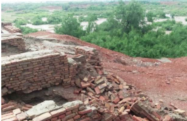
Undermining of wall by run-off, SD area © N. A. Sangha
