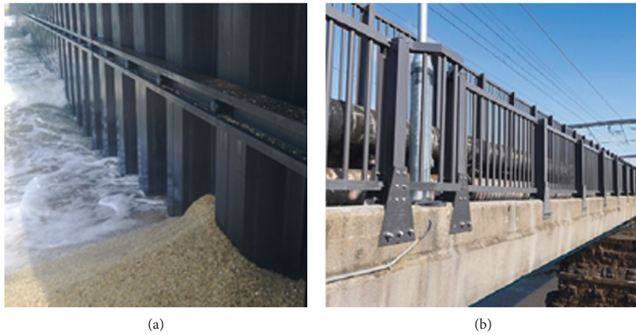
FIGURE 4: Pultruded retaining wall in Azerbaijan (a) and pultruded railway bridge barriers in England (b) [9, 10].
