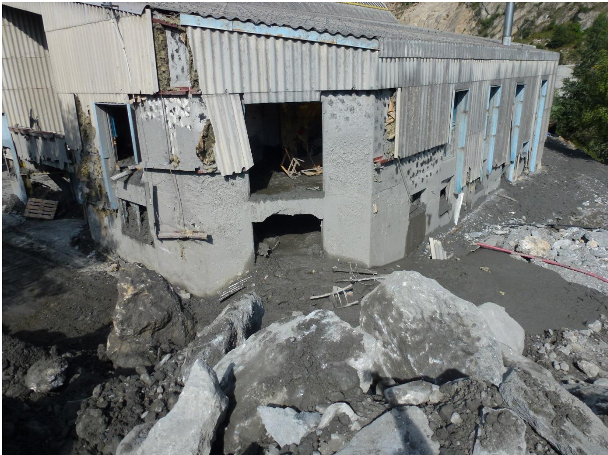
Figure 18 Example of destructive impact of debris flow that overflow its channel banks and spread on alluvial fan (photo G. Piton)
