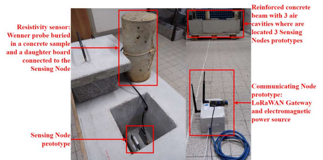
Fig. 6. Photographs of an experimental set-up of Sensing Nodes embedded in a reinforced concrete beam.
