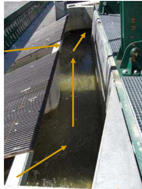
collecting bypass channel
