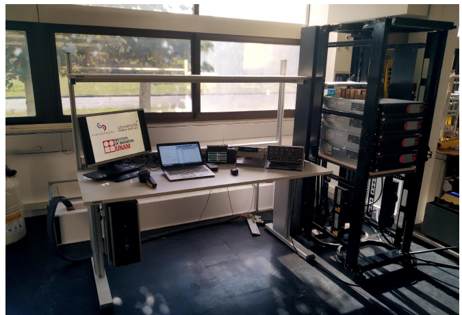
Fig. 1. Overview of the 4800 A Gargantua test station for acquiring the V - I characteristic of HTS power cables at 77.3 K in liquid nitrogen.
