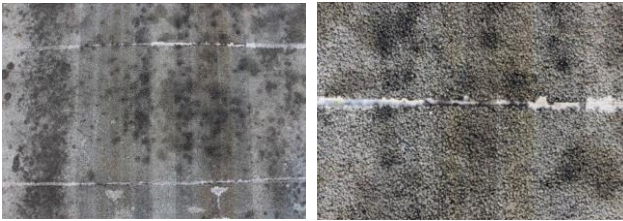
Fig. 8 View of the porous concrete surface, and of one transverse joint at the end of the test
