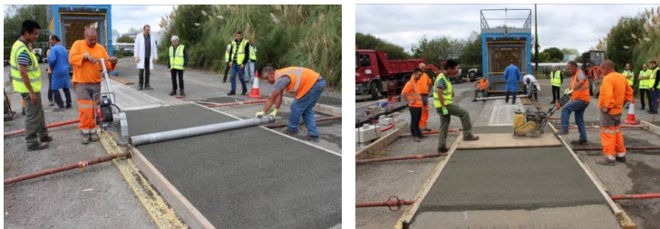
Fig. 5 Compaction of the porous concrete layer with a striker roller, and then a vibrating plate
