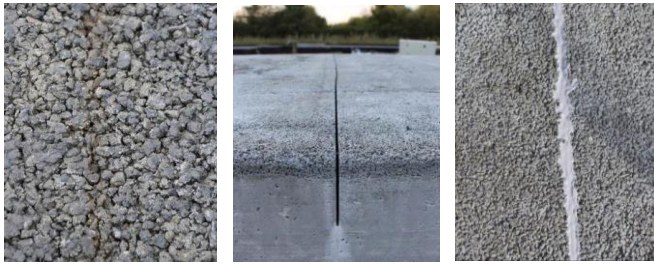
Fig. 6 Surface texture of the porous concrete, sawed joint, and sealing of the joint (Sikaflex resin)
