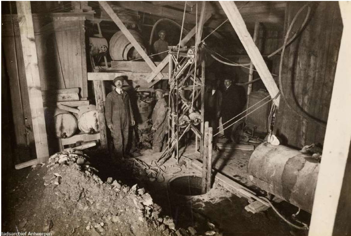
[fig.2] Betonnière et Gun (canon à ciment). Picture of the 'hold' of the ship that was used to hide machinery, dirt and dust from the public space. Source: Felixarchief Antwerpen
