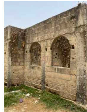
Vacant dwelling, affected by the raising aquifer.
