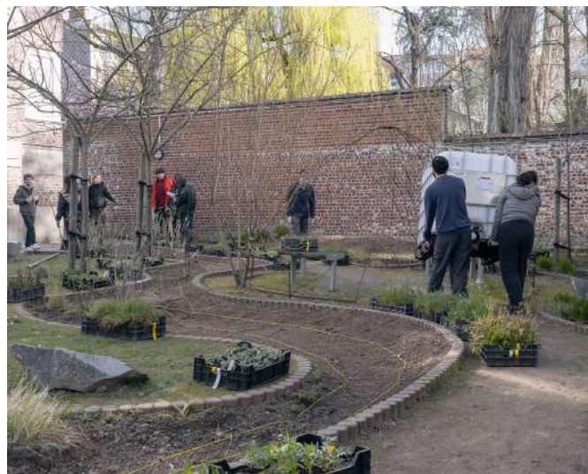
[Fig. 4] The construction site in the collective garden of the social housing of Strauwen: view on the vegetated infiltration basin in the adjacent garden. Source: Bruno Dias Ventura
