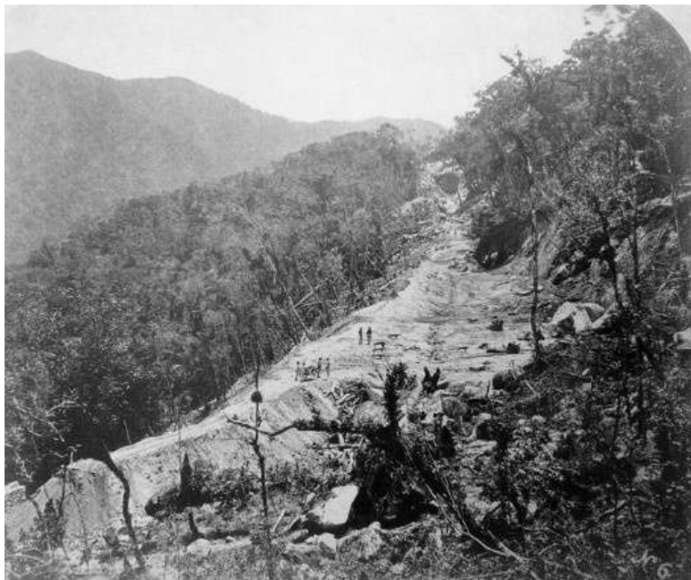
[fig.1] Preparation of the Serra do Mar terrain for the railway track, undated.
