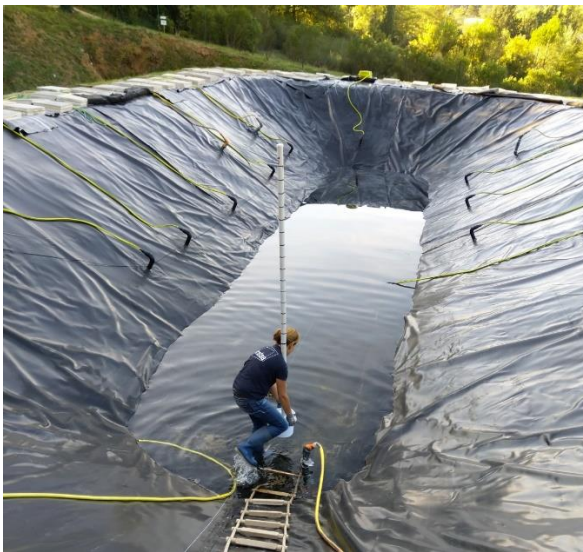
Figure 5. Leaks insertion system.
