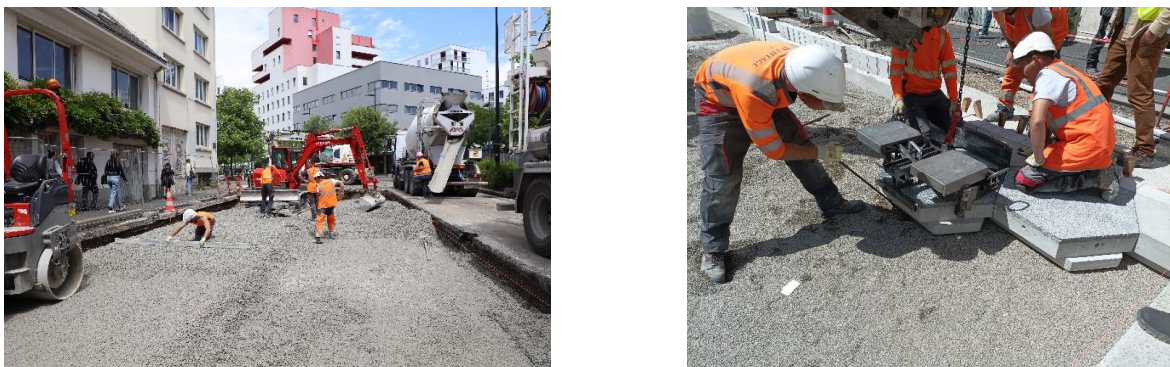
Figure 16 : (Left) Placing of the excavatable porous cement treated aggregate. (Right) insertion of the slab with the handling tool specifically developed
