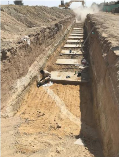
FIGURE 2. View looking south along the border fence in Zone Ab showing the sequence of works, with archaeological investigations and recording of a falaj in the foreground, and in the distance backfilling around the fence foundations.
