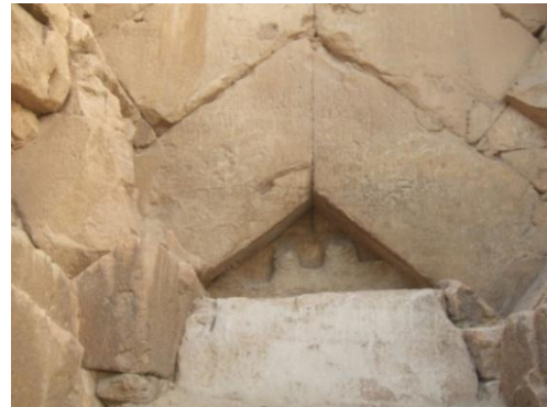
Photo of the Strabo Stone inserted beneath the lower pair of rafters. On the left, the foot of a broken rafter is visible.
