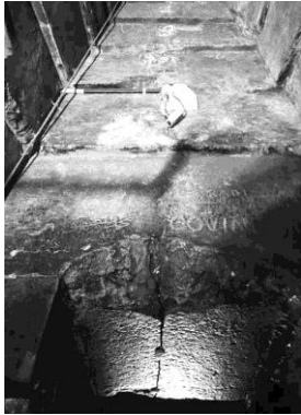
The lintel on the South wall of the Grand Gallery was fractured to remove a block sealing the access corridor to the Portcullis Chamber.
