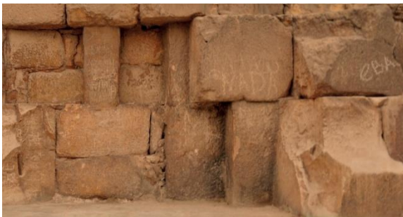
Close-up of the masonry, visibly altered, in the area where the anomaly was detected.
