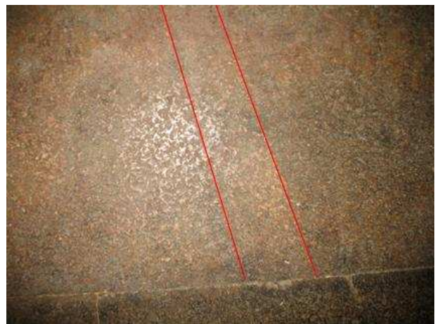
Cracks on the lower part of the lintel
