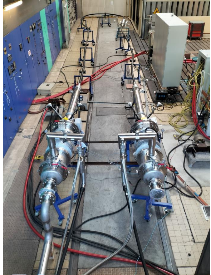
Fig. 12. Cable type test loop installed at the SNCF Railway Test Agency (SNCF-AEF), including two terminations and a joint.
