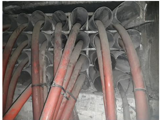
Fig. 3. Existing cable duct bank between the substation and the platform. Each conduit is filled with one 400 mm 2 copper cable (500 A each).
