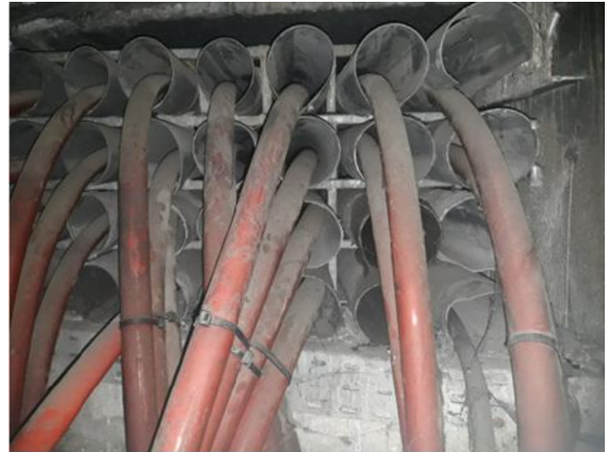
Fig. 3. Existing cable duct bank between the substation and the platform. Each conduit is filled with one 400 mm 2 copper cable (500 A each).
