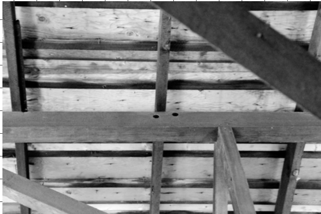
Detail photo of a timber purlin in a barn in New Jersey, 2023. Image courtesy of Erin Besler.
