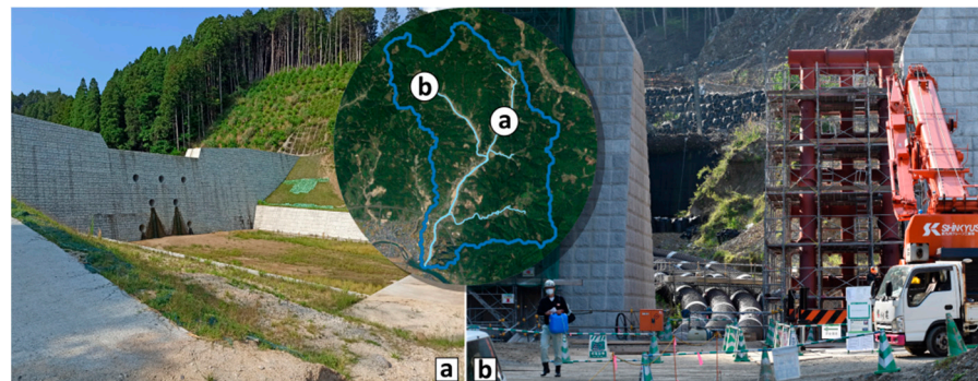
Figure 7. Illustration of the sabo dam constructed in the AK River. (a) Closed-type sabo dam AK16, ©M. Dumont, 2022; (b) slit-type sabo dam OT15-6, ©V. Siccard, 2022.
