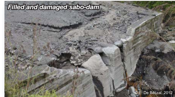
Built in 2010, upstream Apu river, this sabo dam only lasted a few months.
