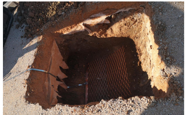
Fig. 4. Grounding point created for the generator in case B.
