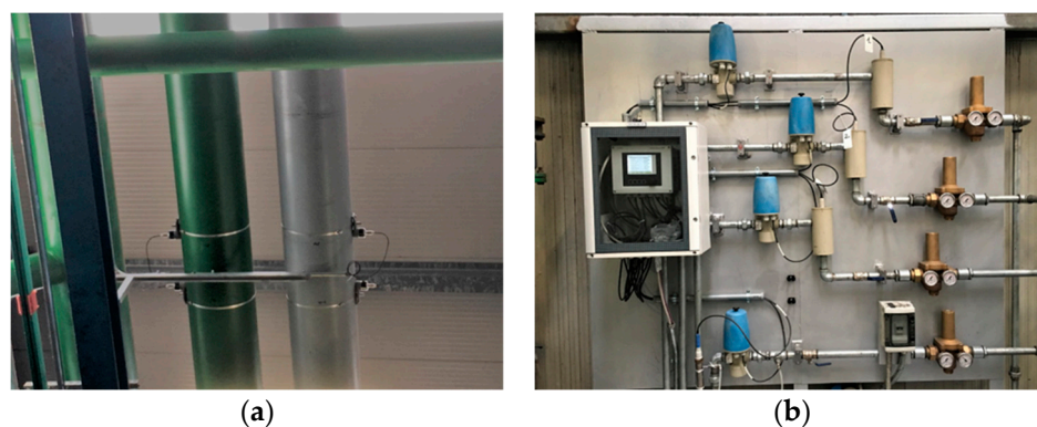
Figure 2. (a) Installed ultrasound flowmeters; (b) electrical conductivity and pH sensors.
