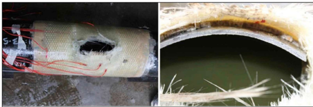
Fig.6. Failure of repaired pipe at repaired/defect region [18].
