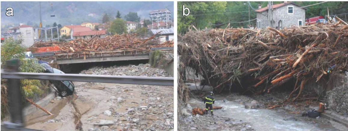
Figure 1: Woody debris accumulations upstream bridges in close vicinity to elements at risk (Lucia et al., 2015).
