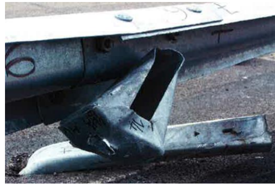
Figure 7 Bolts pull out failure of post - spacer connection [14]
