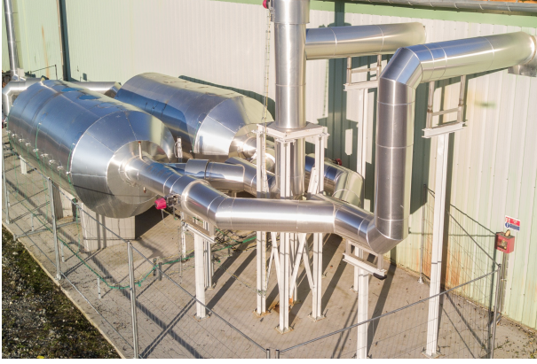
Fig. 1. First industrial scale EcoStock® of 4MWh th at 600 °C developed by ETC.
