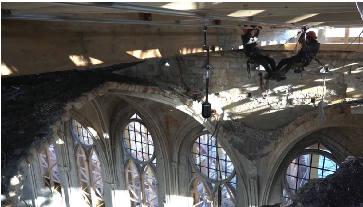
Fig. 2: Rope access technicians moving away from the scanner positioned on one of the rails mounted for the occasion under the technical floor covering the extrados of the vaults of Notre-Dame de Paris. (c) Notre-Dame: building a digital monument, 2020. https://images.cnrs.fr/video/6934 .
