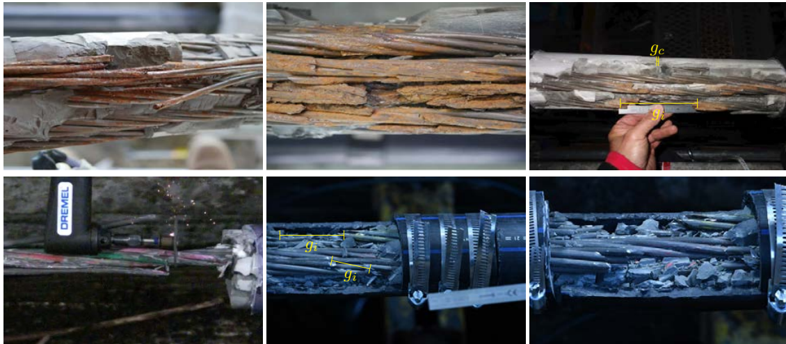
FIGURE 9. Up photos of damage on opened tendon on a bridge © IFFSTAR for Sanef. Down photos of broken wire during the experiments
