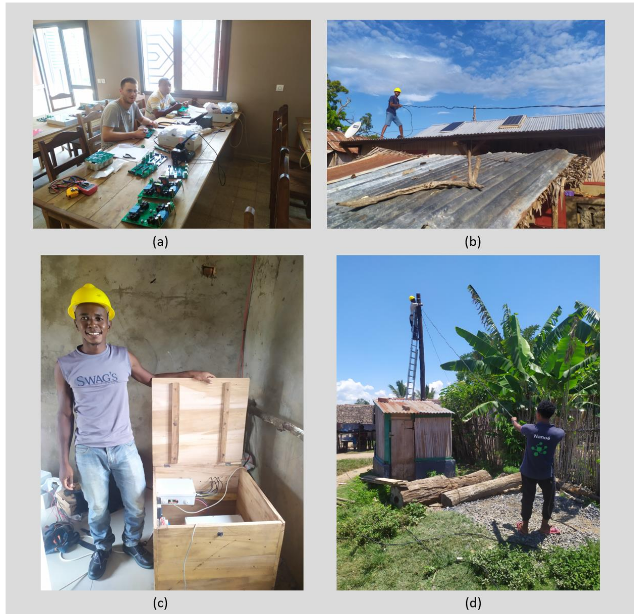
Figure 7: Field installation of Ambohimena microgrid: (a) Assembling of the interconnection modules, (b) Installation of the electric cables, (c) Installation of an interconnection module, (d) Cable connection on an electric pole.
