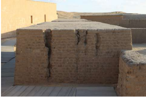
Figure 8: Gullies formed on a recently partially reconstructed entry pylon of one of the tombs of the New Kingdom necropolis at Saqqara.
