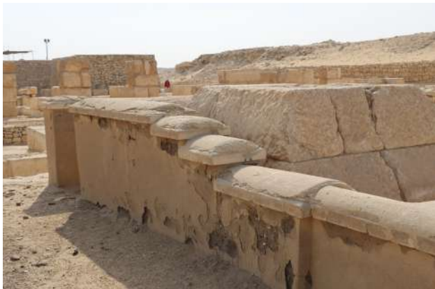
Figure 6: The conservation works (method C) did not prove efficient during the 2020 rains.
