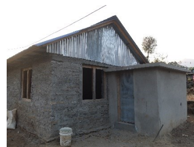
Addition of an extra room, in direct contact with the « core » house. The risk is high of
