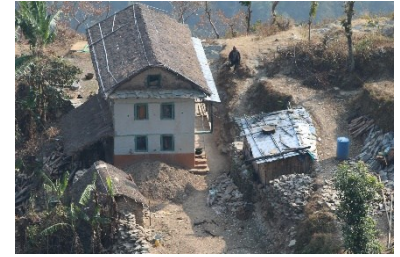
Birds eye view on the layout of the house under reconstruction, ward 6, Bijulikot, Ramechhap –© Wendy van Amerongen
