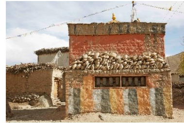
Façade paintings are part of the maintenance practices and cultural identity, Geling, Upper Mustang, 2016 ©Marie Schuiten
