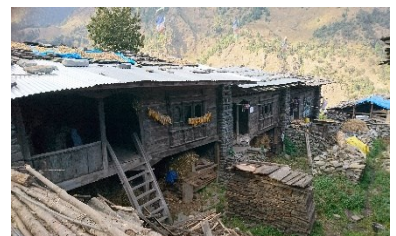
CGI sheets roofing in place of wooden tiles, in cold areas reduces indoor temperatures, Gatlang, Rasuwa –©HRRP
