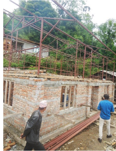
Light steel frame structure for upper storey on BMC ground floor, Jiri, Dolakha, 2017 – ©HRRP
