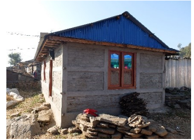
Wooden seismic bands covered with cement plaster: risks of rapid rotting of the timber (due to humidity) with no way to control the state of the timber, Sindhupalchok, 2018 – ©CRAterre
