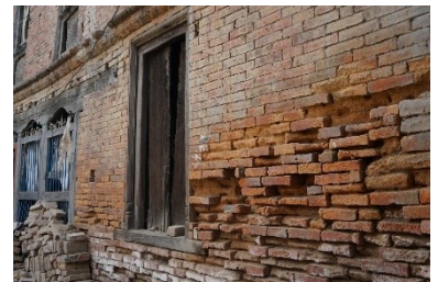
Erosion of bais of burnt bricks due to capillarity/ lack of proper drainage, Bakhtapur, 2016 ©CRAterre
