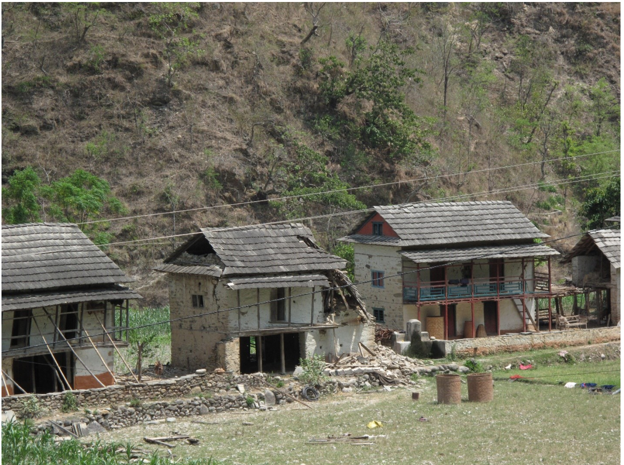
Road from Mantali to Deurali, Ramechhap. on the same plot, with the same local building materials, a series of neighbouring houses suffered very different damage, most likely due to construction details and maintenance. 2015 ©CRAterre
