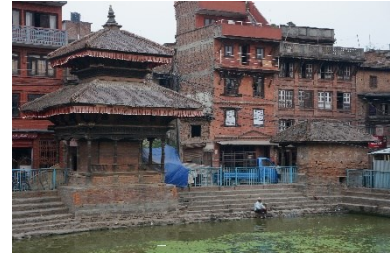
“Fake” traditional “Newari façade- the façade is “plugged on a Brick masonry and RCC frame building, Bhaktapur, 2016 ©CRAterre
