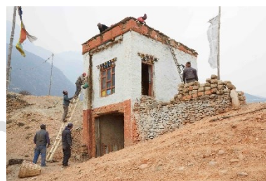
Roof maintenance, adobe house with clay plasters /paints. Drakmar, Upper Mustang 2016 – ©Marie Schuiten
