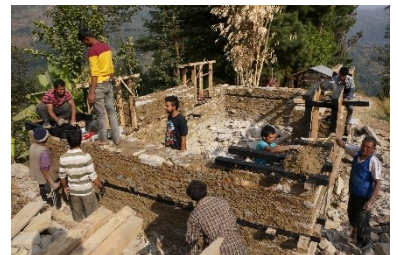
Training for masons, under engineers supervision: in a large proportion, men benefit from these opportunities, 2017, Dolakha– ©CRATERre
