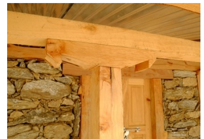
Capital for the support of timber beams, allows lateral displacements without structural disorder, Dolakha, 2105– CRAterre©
