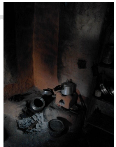
Effects of smoke on the interior walls of a kitchen, where firewood is used on an open fire, with no chimney to vent the smoke– ©CRATERre
