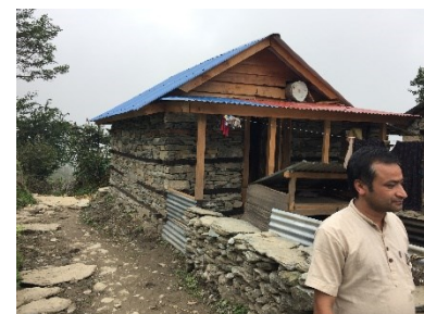
Clear dissociation of roof and veranda for better roof behaviour in case of strong winds, Dadhing 2018 –©HRRP
