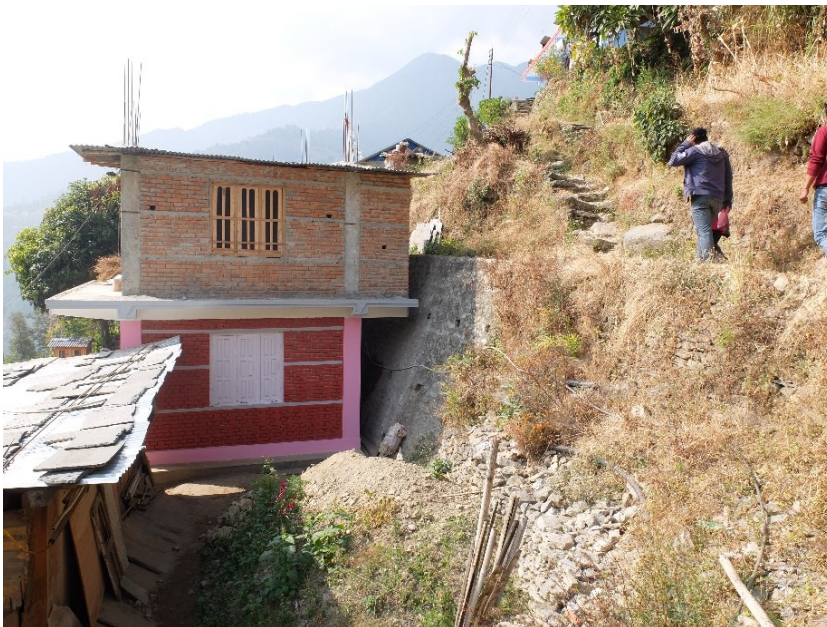
Hazardous vertical extension, asymmetrical load descent, exposed rebar on the roof (probably for future extension), Sindhupalchok, 2018 — ©CRAterre
