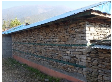
Wind protection. Roof structure is anchored in the heavy masonry walls— CRAterre©
