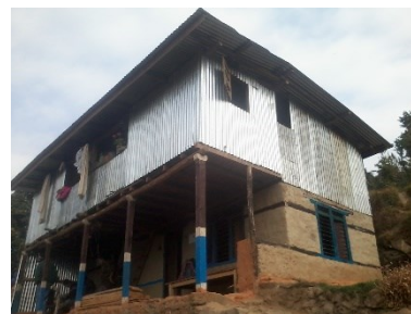
Sound hybrid structure: masonry ground floor & timber+ CGI sheets storey, Bhojpur. ©HRRP
