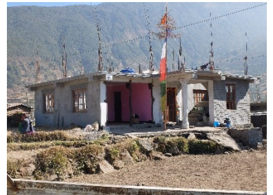
Rebars left “nude” for future vertical extension: high risk of corrosion before they are embedded in concrete columns. Sindhupalchok, 2018. – ©CRAterre
