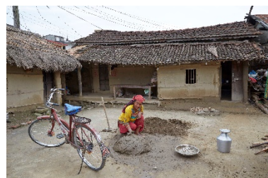
Artisan preparing mud mortar for regular maintenance of the plasters, Mithali village near Janakpur, 2016– ©Marie Schuiten
