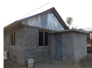
Addition of an extra room, in direct contact with the « core » house. The risk is high of damages, in case of earthquake – ©HRRP
