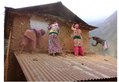
Owner driven retrofitting of damaged SMM houses. Women providing the preparatory work, the skilled / paid tasks being left to men, Dadaputalibazar, 2019– ©HRRP
