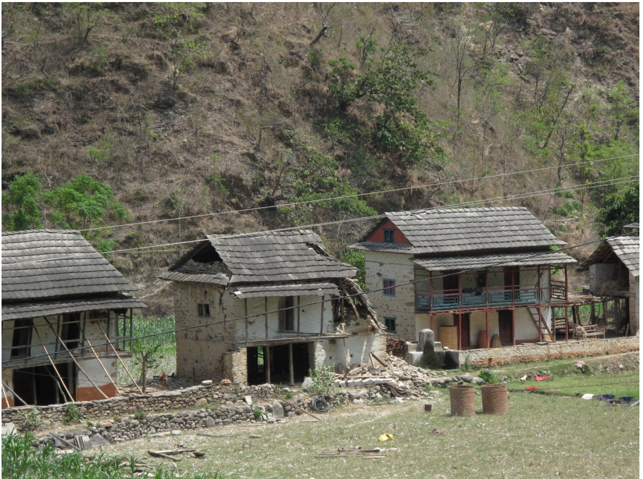
Road from Mantali to Deurali, Ramechhap. on the same plot, with the same local building materials, a series of neighbouring houses suffered very different damage, most likely due to construction details and maintenance. 2015 ©CRAterre
