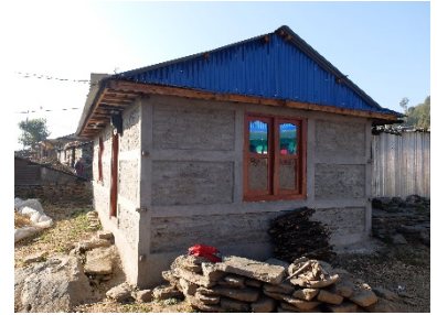
Wooden seismic bands covered with cement plaster: risks of rapid rotting of the timber (due to humidity) with no way to control the state of the timber, Sindhupalchok, 2018 – ©CRAterre
