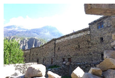
Settlement in the village of Manang. Minimum openings in massive stone walls, 2013– ©Mathilde Chamodot
