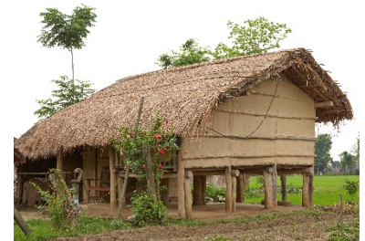
Cross ventilation, bottom ventilation and thick fiber roofing regulate the indoor humidity and temperature , Tharu village, Terai, 2016– ©Marie Schuiten
