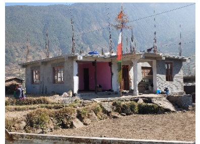
Rebars left “nude” for future vertical extension: high risk of corrosion before they are embedded in concrete columns. Sindhupalchok, 2018. – ©CRAterre
