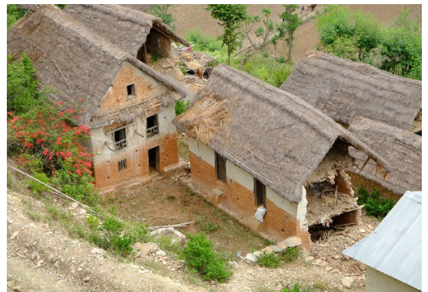
Stone in mud mortar EQ affected houses, Dolakha, 2015 – ©CRAterre
