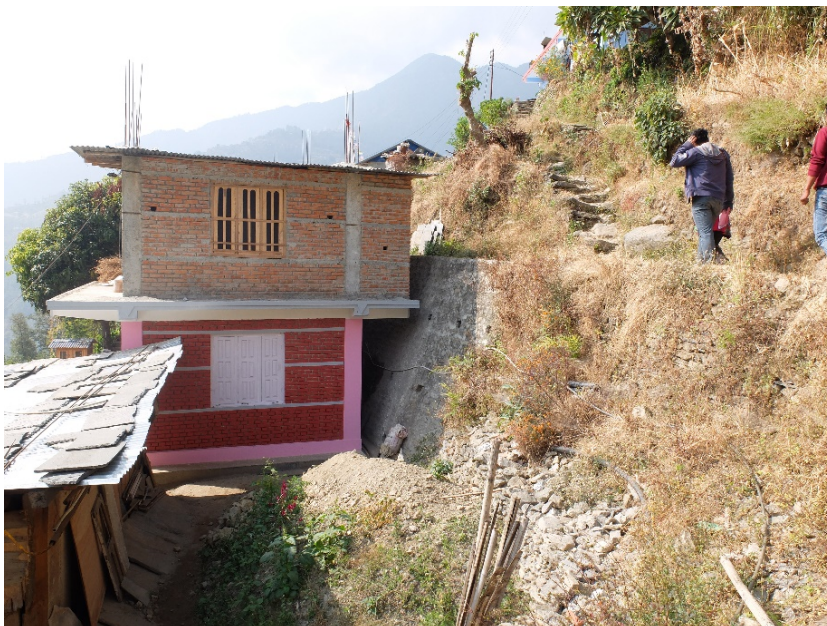
Hazardous vertical extension, asymmetrical load descent, exposed rebar on the roof (probably for future extension), Sindhupalchok, 2018 – ©CRAterre
