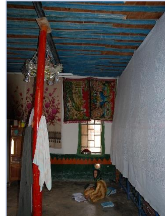
Intermediary metal I-beam to support joists for bigger width of room – © CRAterre
