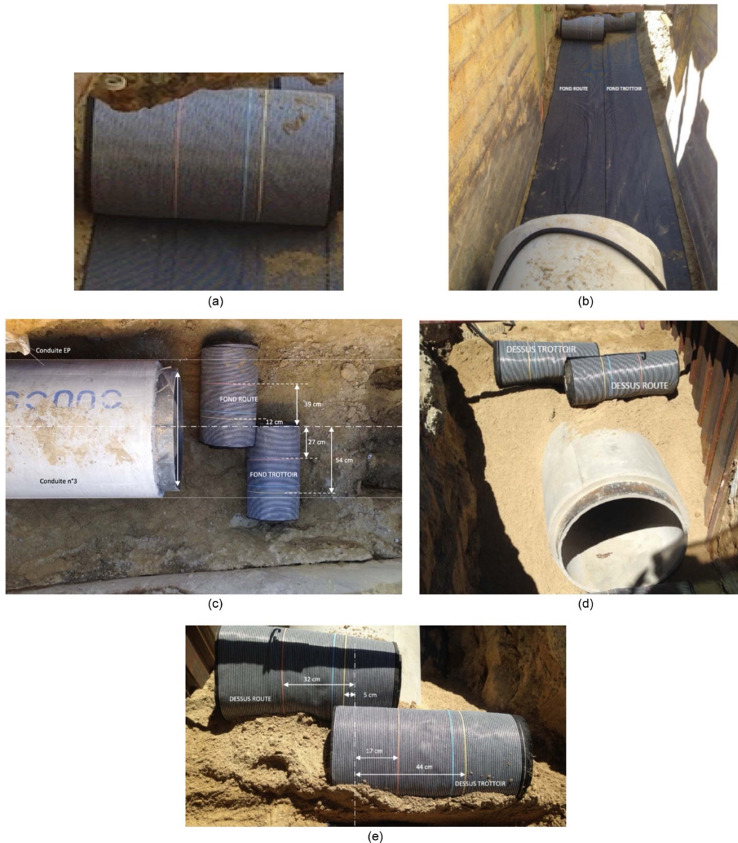
Fig. 2. Sensor-enabled geotextile and its location ( FOND means below, DESSUS means above, ROUTE means roadside, and TROTTOIR means sidewalk side): (a) sensor-enabled geotextile; (b) sensor below the pipeline; (c) location of measuring-loop optical cables (below the pipeline); (d) sensor above the pipeline; and (e) location of measuring-loop optical cables (above the pipeline).
