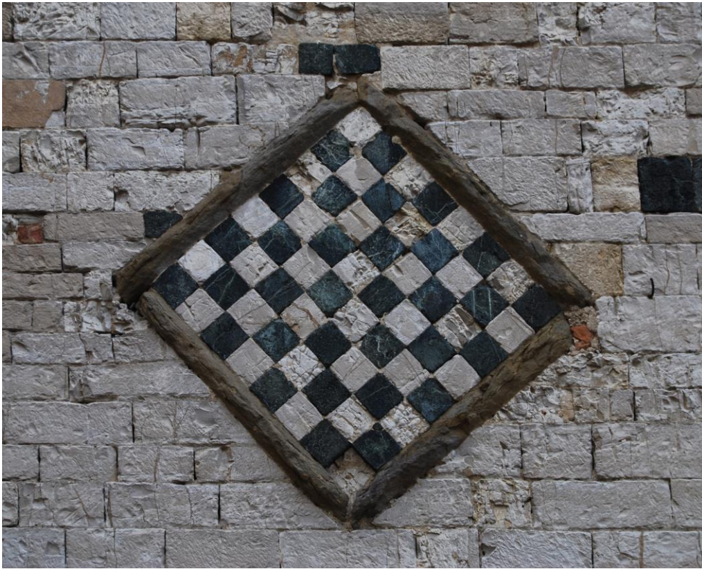
Figure 4 - Chessboard composed of sketches of Green Marble from Monte Calvi and Pietra Alberese present on the north elevation of the Pieve di Sant'Agata del Mugello.
