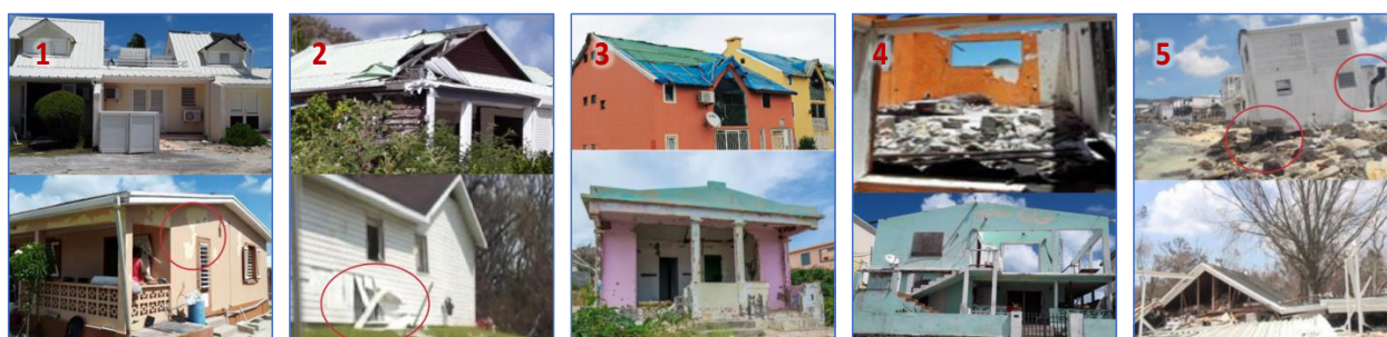
Figure 4. Different damage classes of residential buildings in St. Martin. Classe 1. No or limited damage (hardly visible from the outside/superficial damage to roof, windows, doors, or walls). Classe 2. Minor damage (roof affected in a few places, a few windows or doors broken/exterior walls partly in need of repair). Classe 3. Moderate damage (roof affected in many places, almost all windows or doors broken/cracks in walls are repairable). Classe 4. Severe damage (+50% of roof ripped off and structural damage/windows or doors completely broken/load-bearing walls severely damaged but not destroyed). Classe 5. Destroyed (foundations destroyed/roof structure and load-bearing walls totally destroyed).
