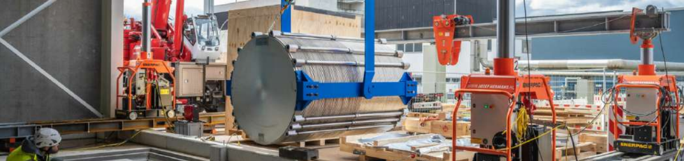
Arrival of the first electrolyser modules RWE 10 MW ALK green hydrogen facility in Lingen, Germany (April 2023, Courtesy of RWE)
