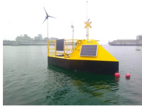
Fig. 3: Fixed beacon hosting the UWA transmission system.
